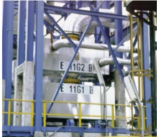
Two out of totally four horizontally mounted Compabloc in titanium used for vapour condensing in the atmospheric distillation tower.
